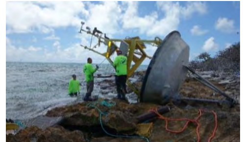
Salvage technicians dismantle the buoy tower prior to removal. Photo: Sea Engineering, Inc.
