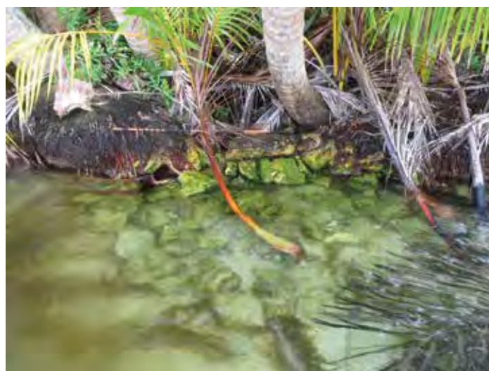
Figure 88: Slabs of cut beach rock emerge from beneath the perimeter tree growth, near the former pier (location different from cut rock slabs on the lagoon noted by the terrestrial team).
