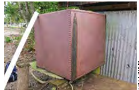
Figure 194: Ship tanks #1 (Tualaga Village) in-use.
