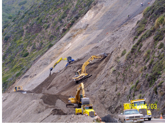
Crews managed by Caltrans clear debris from the 2011 Alder Creek Slide. Caltrans and MBNMS work together to minimize the impacts of debris deposition.
